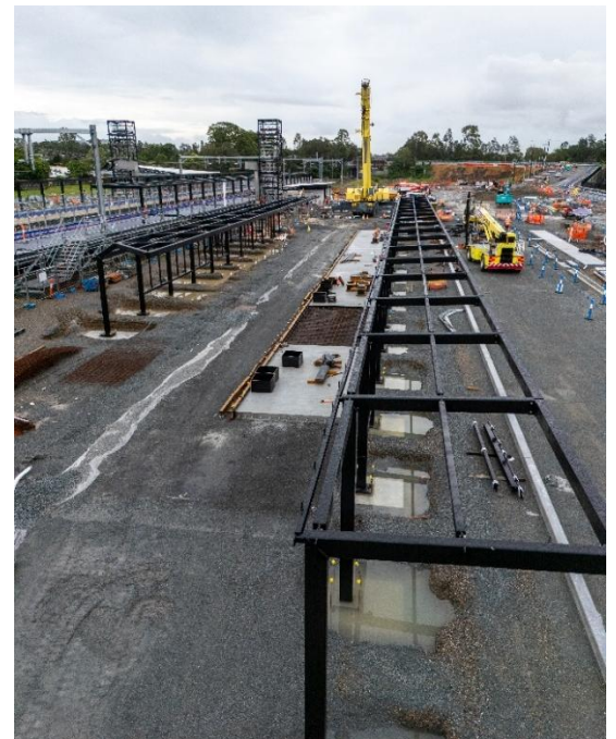
Above: Kiss 'n' ride, taxi bays and new bus stop shelter steel installation
