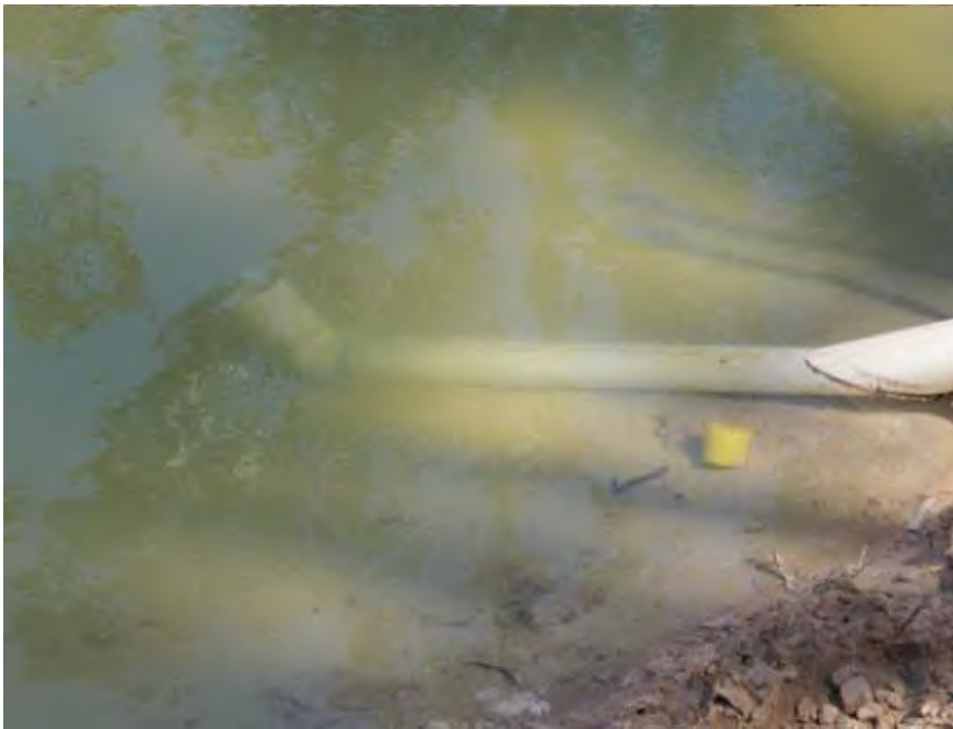
Ensure inlet is positioned above settled solids to stop sediment being sucked into the pipe
